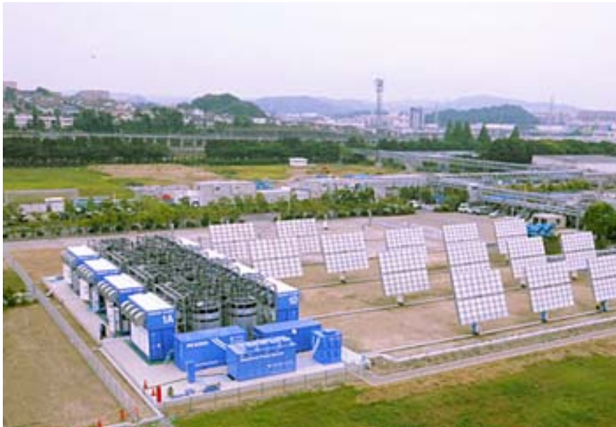
Vanadium 1 MW x 5 hr flow battery installed at a PV farm (Sumitomo Electric)
